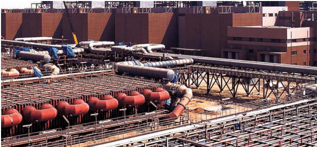
Desalination Plant (Resource : Doo San heavy industries)
