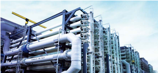
RO desalination plant
